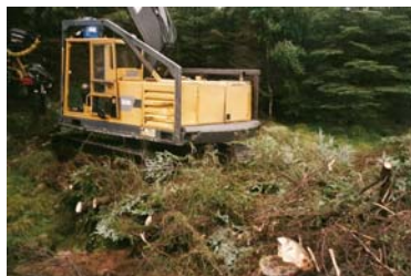
Figure 6. Harvesting at Dromalohurt using a temporary bridge made from log and brush to facilitate the harvester crossing the stream.
